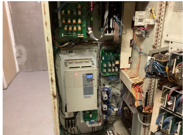
Traction elevator controls
