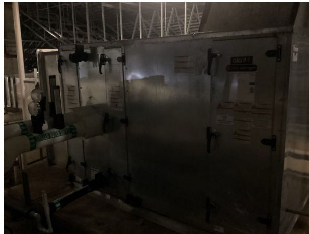
Make-up air unit
