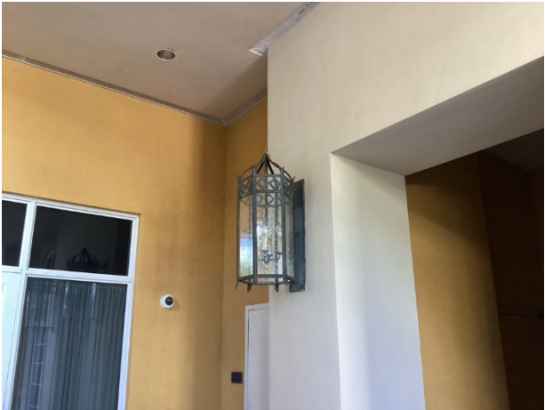
Exterior light fixture
