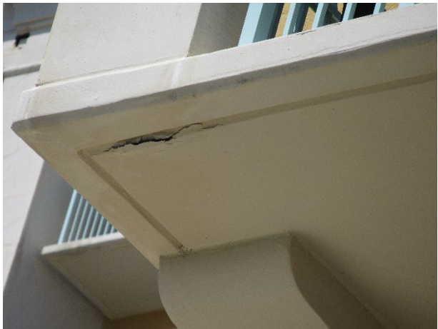
Concrete cracks at balcony underside
