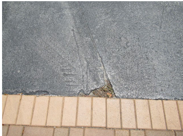
Asphalt pavement edge deterioration
