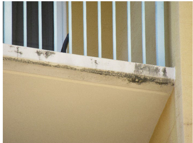
Water stains at balcony underside
