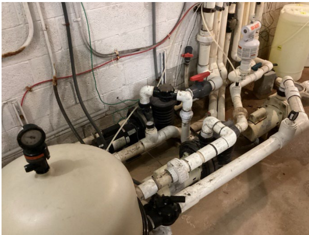
Pool mechanical equipment
