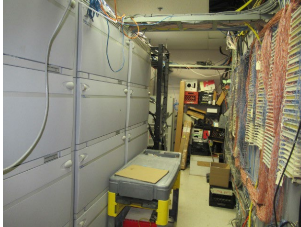
Recently installed telephone system controls
