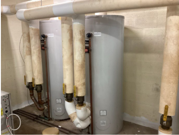
Hot water storage tank
