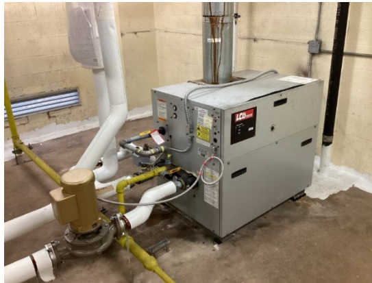
Gas-fired domestic water boiler
