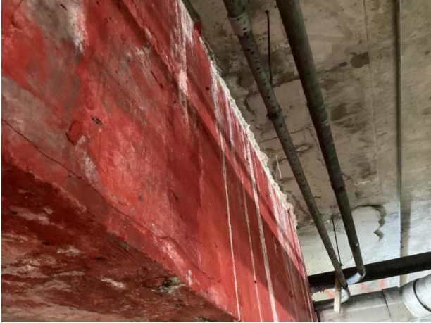
Efflorescence at spa jacuzzi underside
