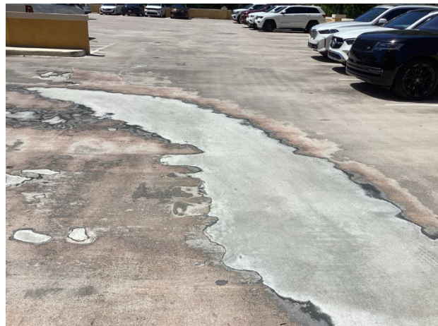
Traffic coating delamination
