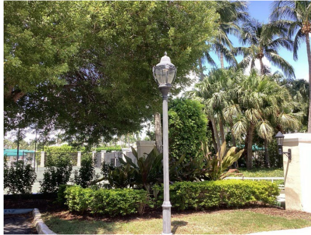
Light pole and fixture
