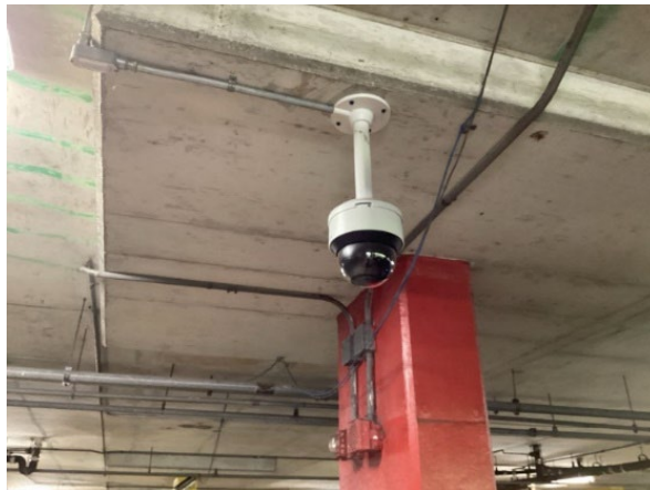
Security system camera
