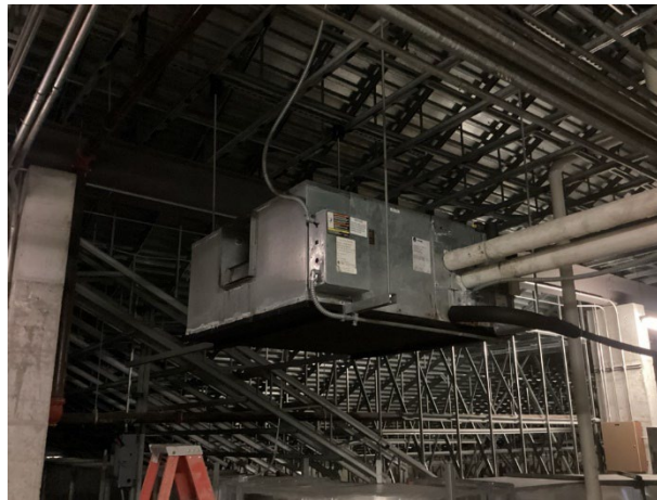
Air handling unit
