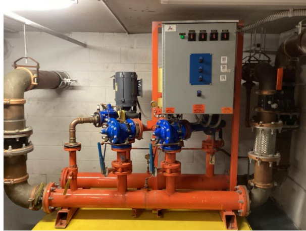
Domestic water pumps
