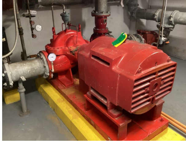
Fire suppression pump
