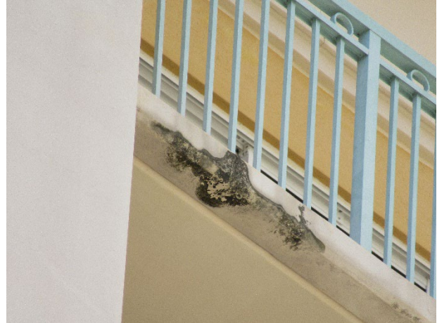
Concrete spall at balcony underside
