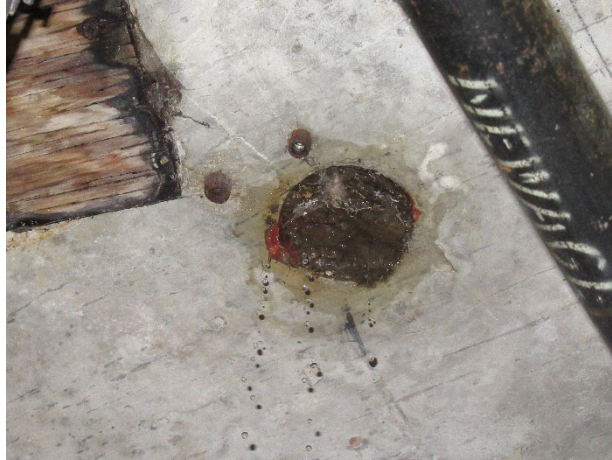
Active leaks underneath men's spa showers
