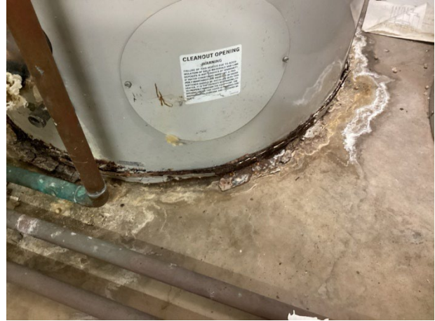
Rust at tank base
