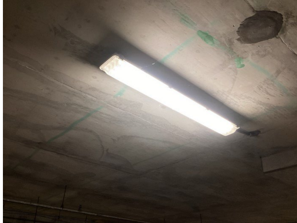
Garage light fixture
