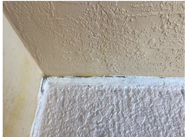
Edge sealant deterioration
