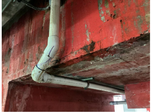
Concrete cracks with active leaks and stalactites at spa jacuzzi underside
