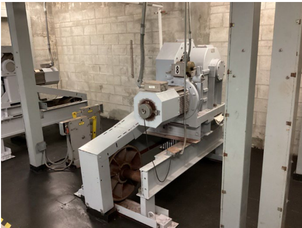
Traction elevator hoists and motors
