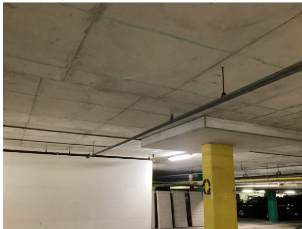
Fire suppression system
