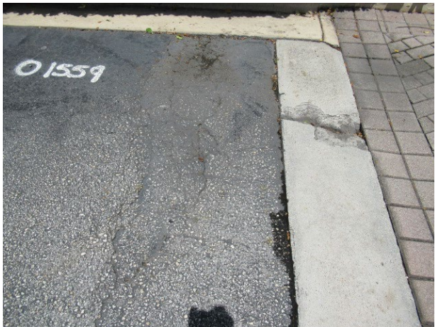
Asphalt pavement cracks
